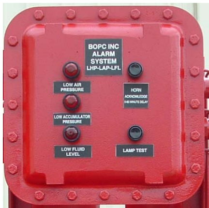
Unit Mounted Alarm Panel
