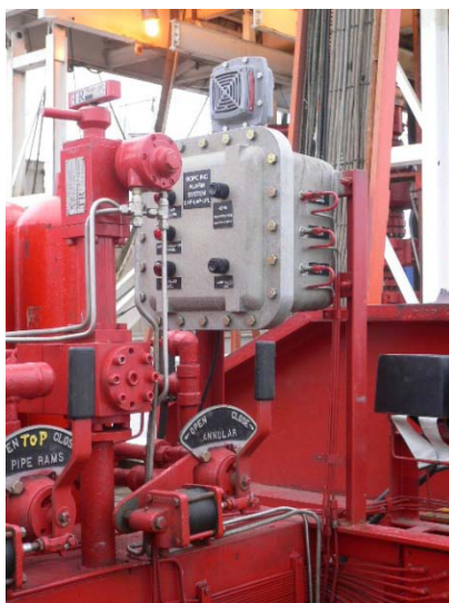
Field installed Alarm System
